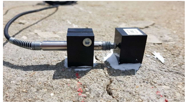
Solartron gauging probe monitoring a crack
